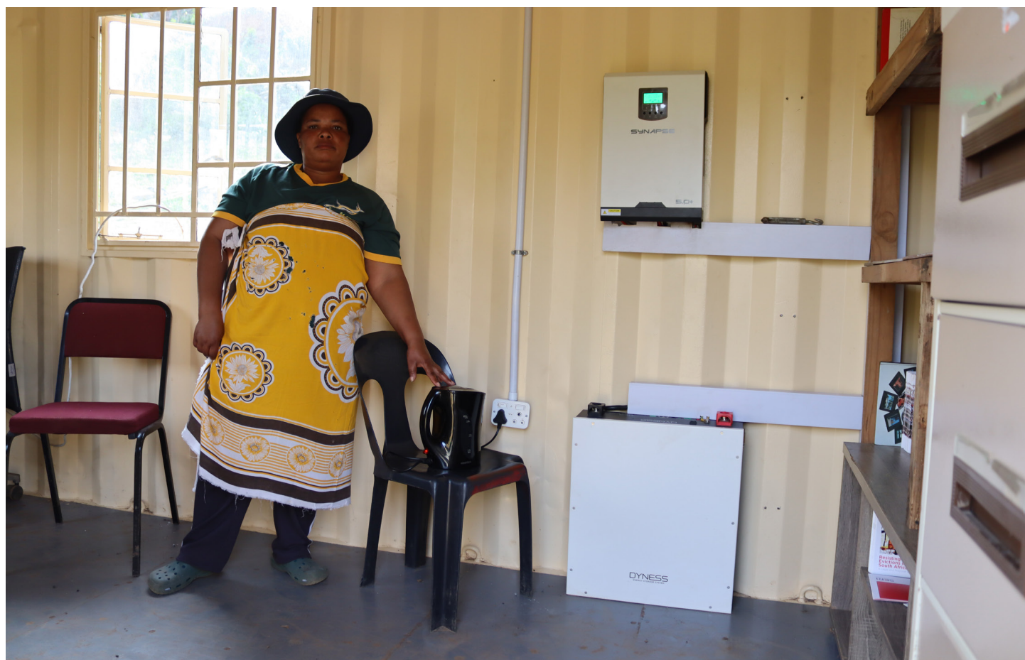
Opposite: The UMIED renewable energy units at Khenana informal settlement in Durban
